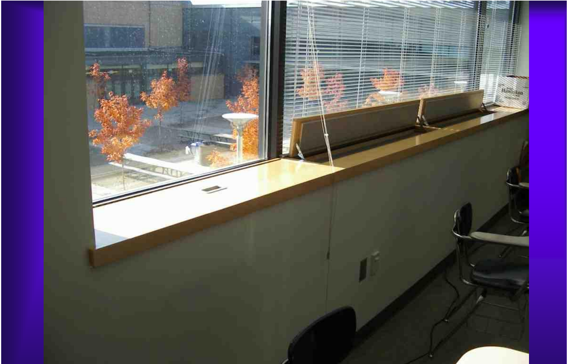
Classroom Passive Air Intake
