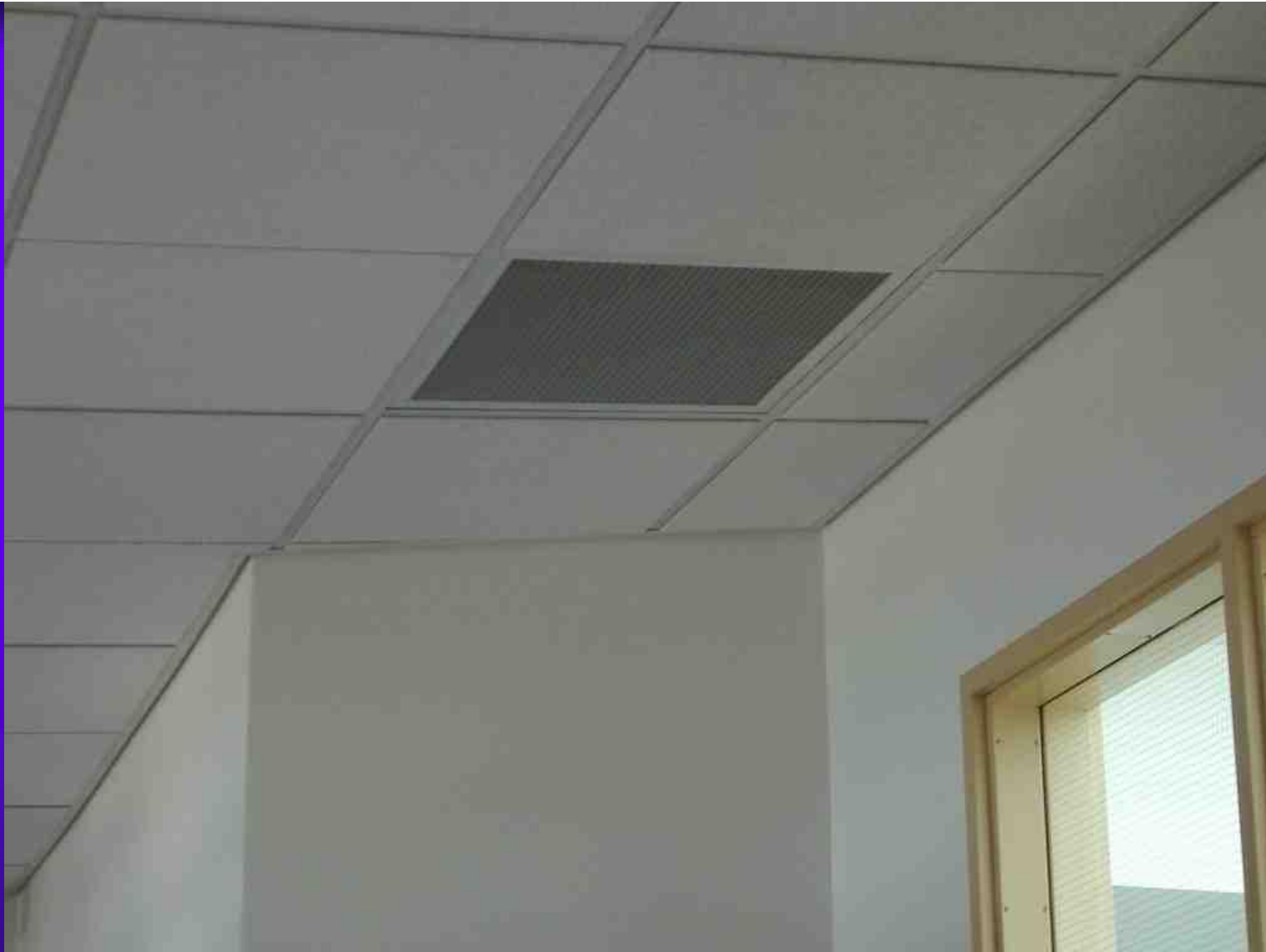
2nd Floor Classroom Passive Return
