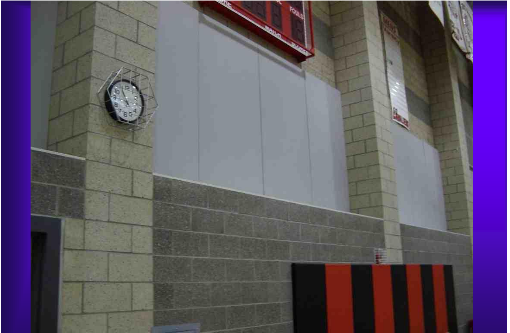
Passive Air Intake Gym (above hallway ceiling)
