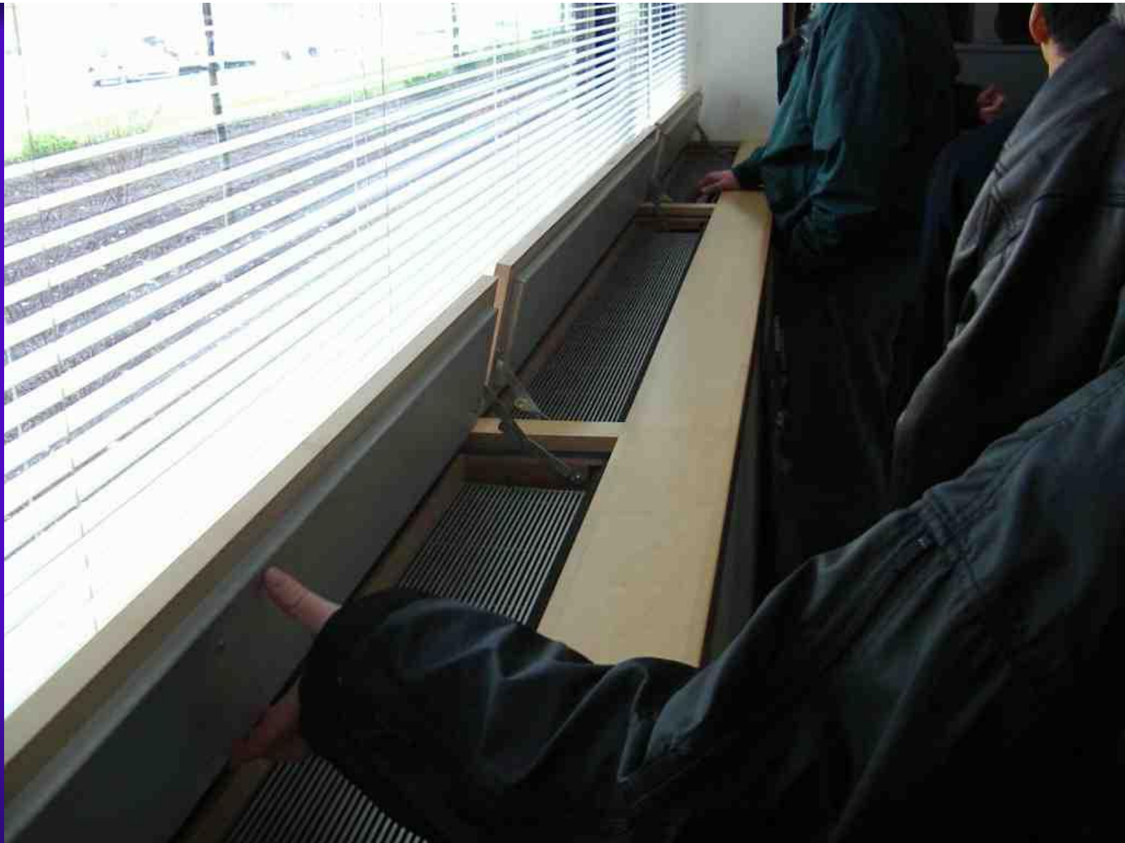
Close-up of Passive Air Intake Classroom
