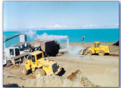
Cold Bay thermal desorption unit
