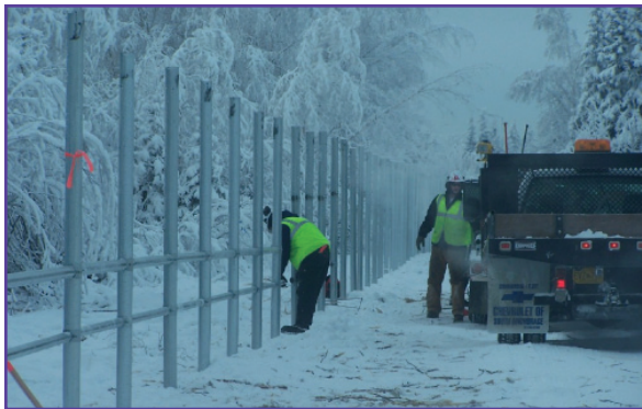
BCS workers building a 16.1-mile boundary fence, designed for arctic conditions, at Fort Wainwright.
